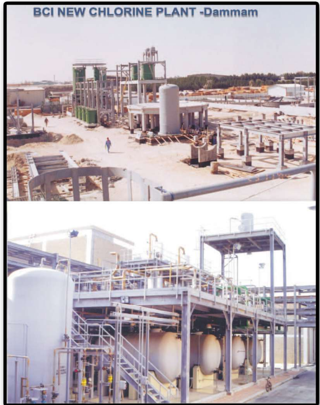
BCI NEW CHLORINE PLANT 2005 1st INDUSTRIAL CITY – DAMMAM
