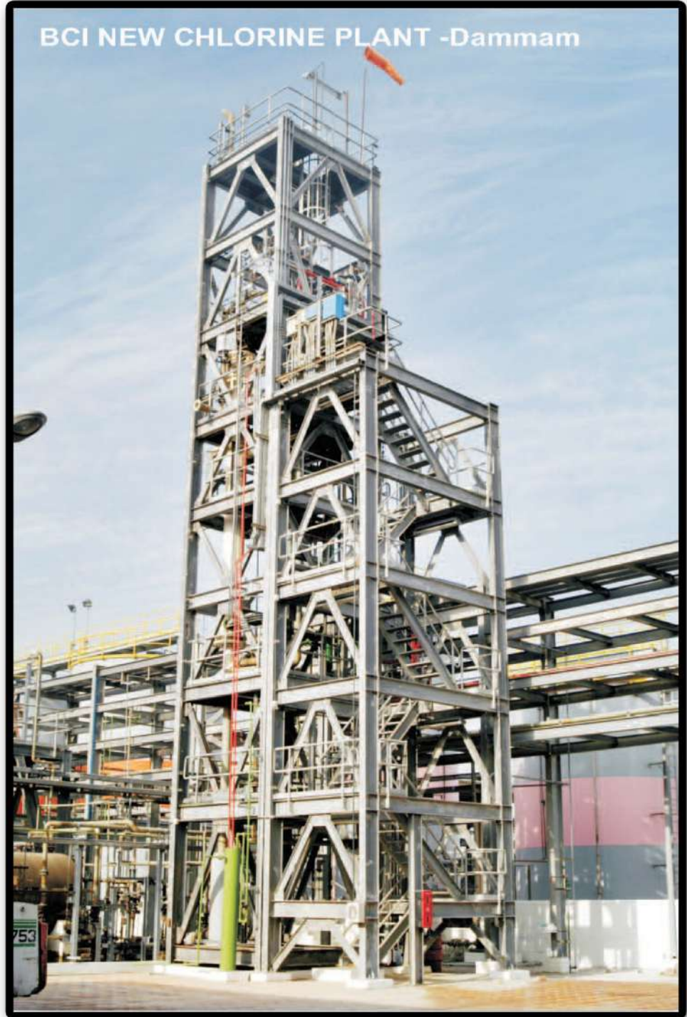
BCI NEW CHLORINE PLANT 2005 1st INDUSTRIAL CITY – DAMMAM
